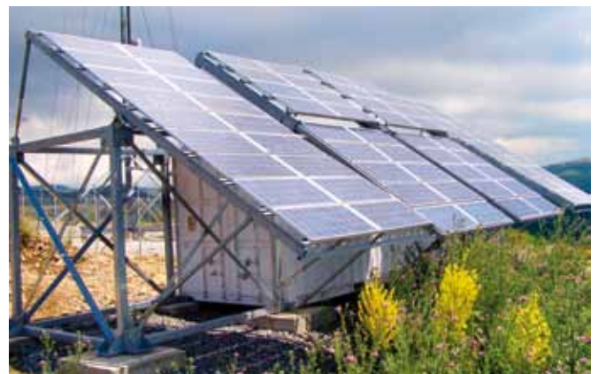
Photovoltaics at GLOBUL base station
